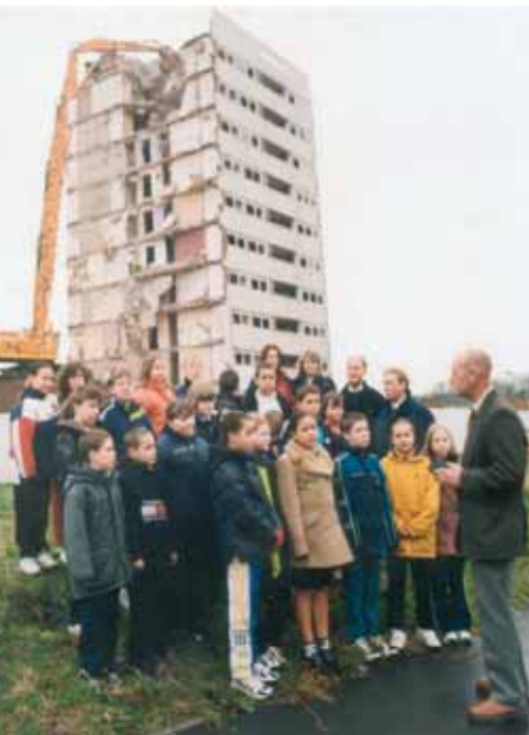
Demolition contractors talk pupils of Chivenor Junior School through the demolition of a tower block on Farnborough Road.
