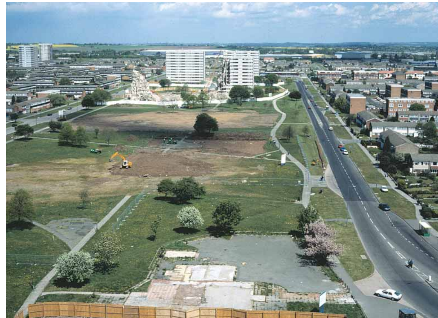
View of demolition of the last four of the Centre 8 tower blocks from Albert Shaw House, c1996. The area in the foreground was replaced by Eden Court Doctor’s surgery and the Sanctuary healthy living centre.
