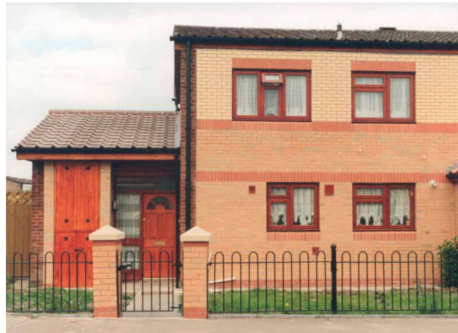
Over 1,300 homes were refurbished to high a specification, bringing them up to modern standards.
