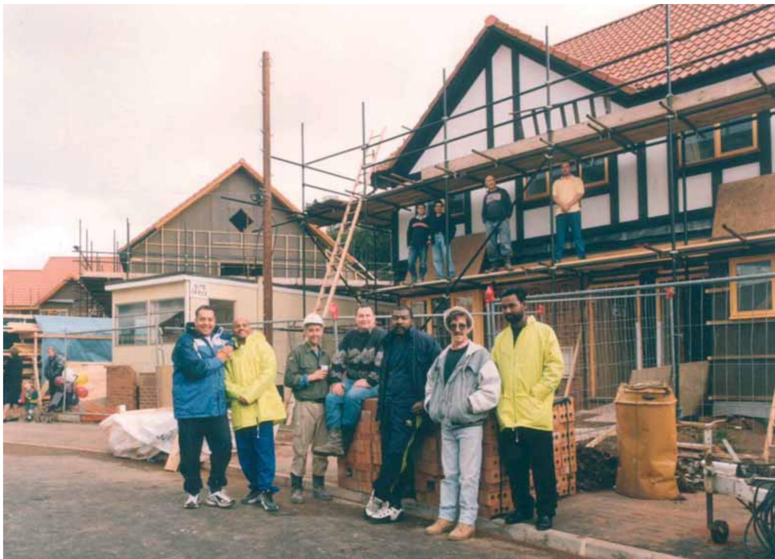
Self-builders take a rest from the construction of 14 new mock-Tudor style homes.
